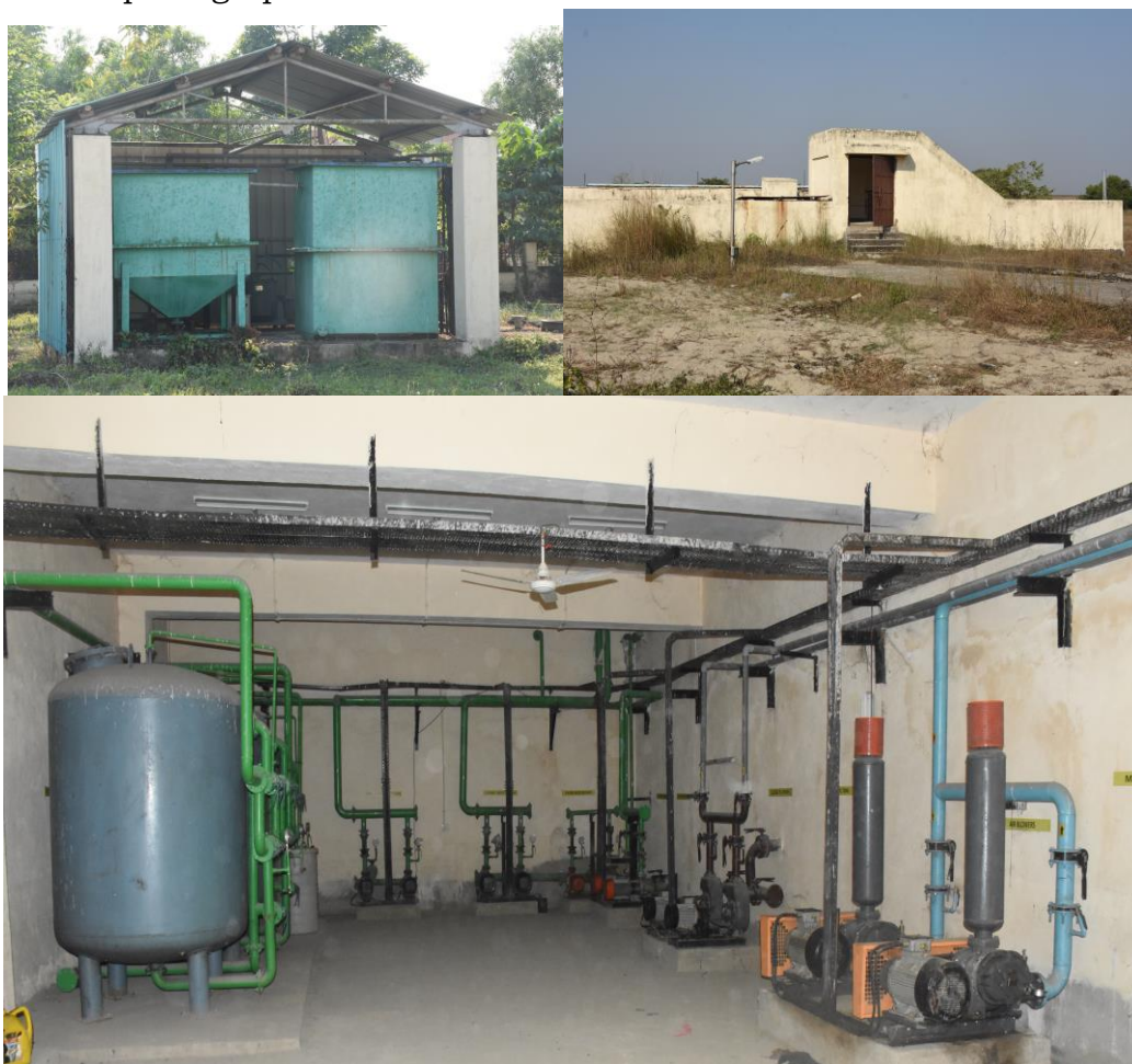
Fig. 5: Biological Waste Disposal and Sewage Treatment Plant
